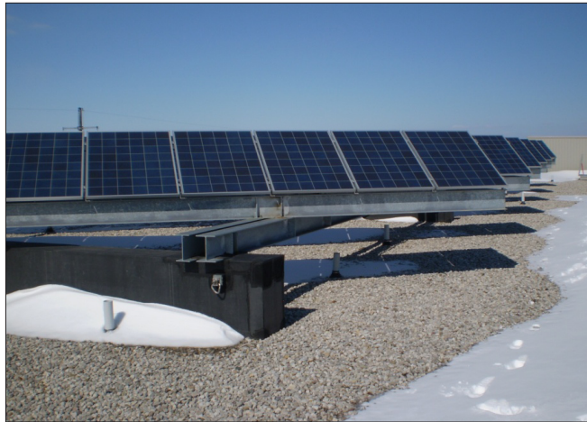
Solar Photovoltaic Array
